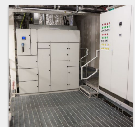
Monitoring of heating, ventilation and air conditioning systems
